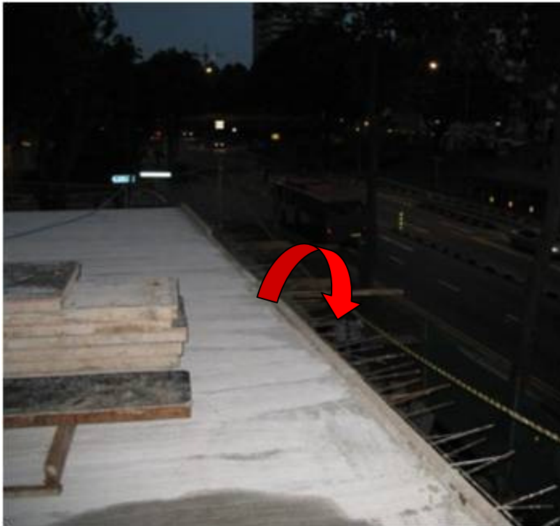
Open edge of building under construction without proper barricades
