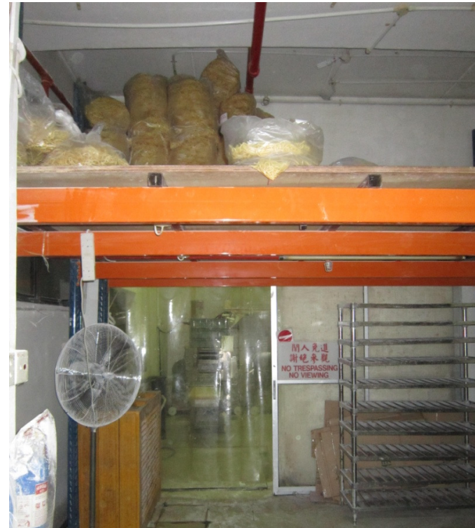
Open edge of mezzanine floor without proper barricades
