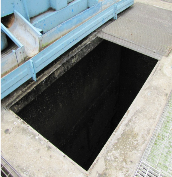
Floor opening created by grating removed
