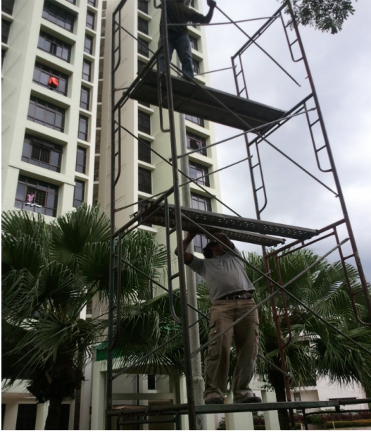
Scaffold without proper guardrails and access
